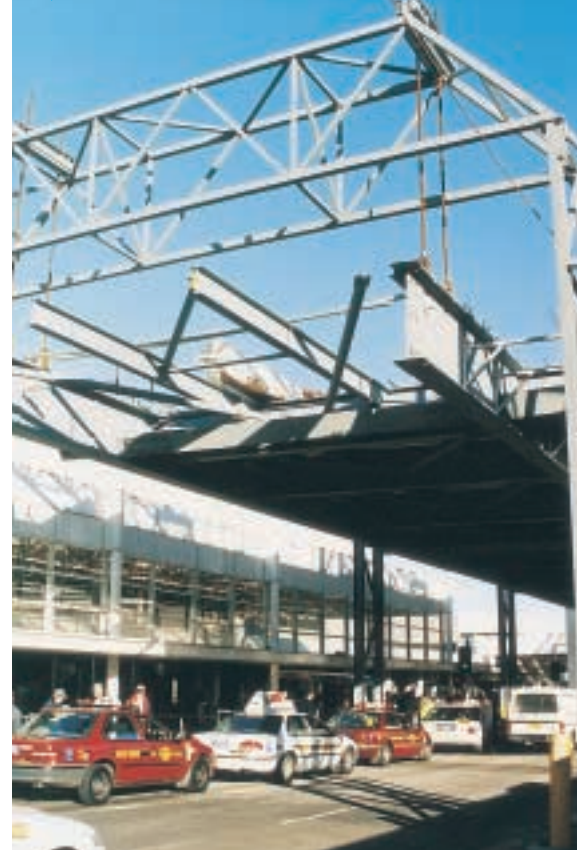
Construction of the elevated roadway was achieved with minimal disruption to traffic below.
