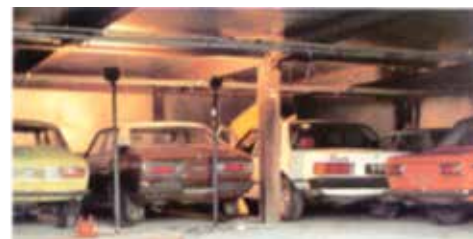
The structure after the fire test
